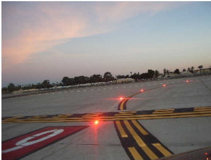
FIG 2-1-12 Runway Entrance Lights
