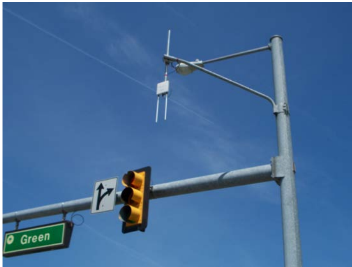
Figure 2: Example of Dedicated Short-Range Communications Roadside Unit Installed at Signalized Intersection
