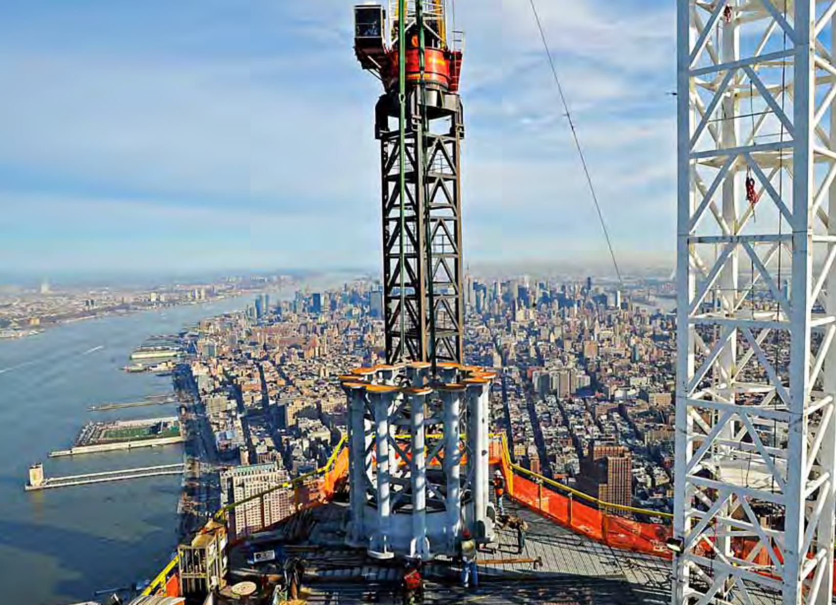
The final two sections of the 408-foot steel spire that crowns One World Trade Center were hoisted into place in May 2013.
