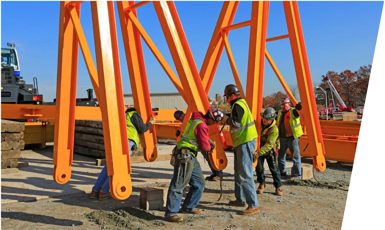
The Bayonne Bridge project marks the first time in agency history that engineers are constructing a bridge roadway deck above an existing one while traffic continues to flow.
