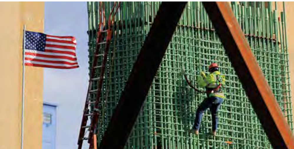
The Goethals Bridge Replacement Project currently fields 35 apprentices working in eight different trades.
