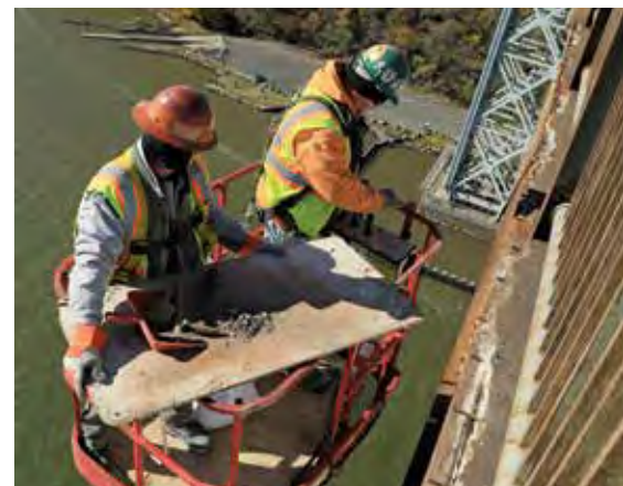
The $82 million state-of-good-repair upper-level steel deck replacement will extend the bridge’s roadway deck life by 15 to 20 years.
