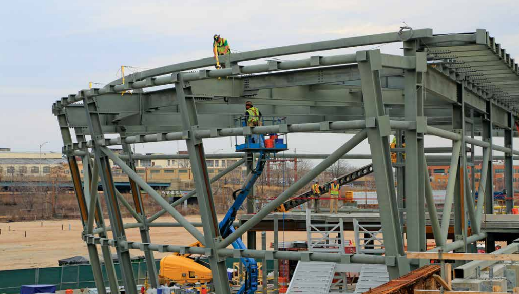
The new Harrison PATH station, a $256 million reconstruction, features glass-and-steel design and fully modernized amenities.
