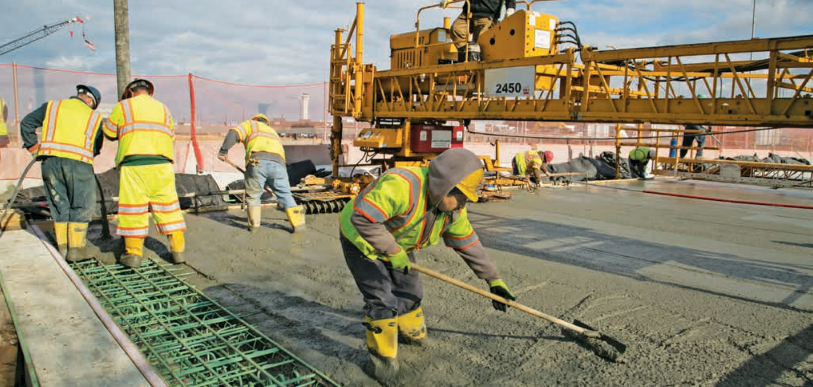
Construction progresses on roadway bridges at Newark Liberty International Airport, designed to reduce congestion and connect the airport's central roadway network to a new Terminal A.
