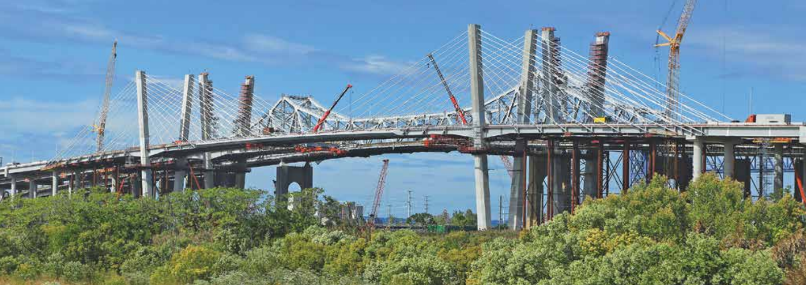
The eastbound span of the new Goethals Bridge opened to traffic in both directions as construction continued on the westbound span.
