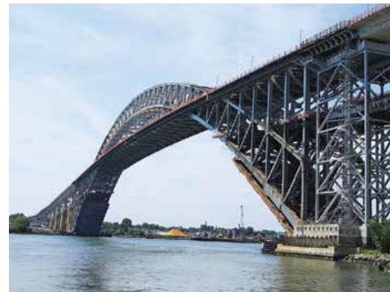
Construction proceeds at the Bayonne Bridge after achieving navigational clearance of 215 feet.
