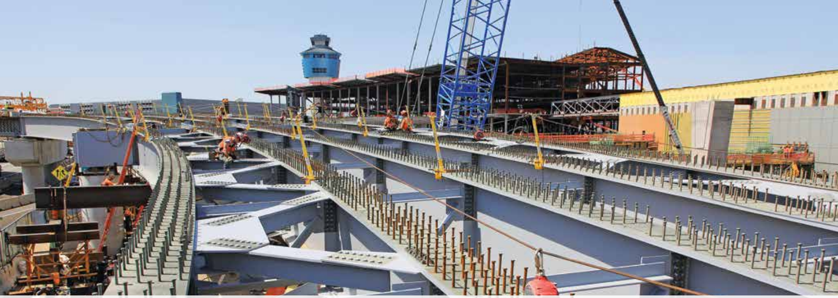
Construction of a new airport roadway system to service the redeveloped LaGuardia Airport.
