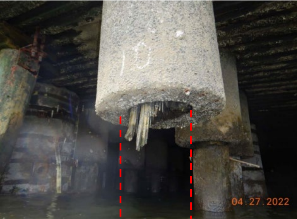
Broken/Missing Pile, Wharf 76
