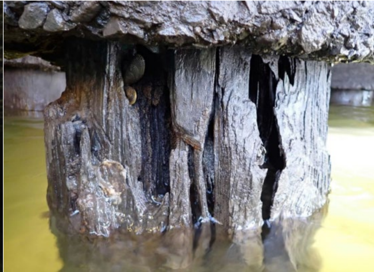
Severely Deteriorated Timber Pile, Wharf 59
