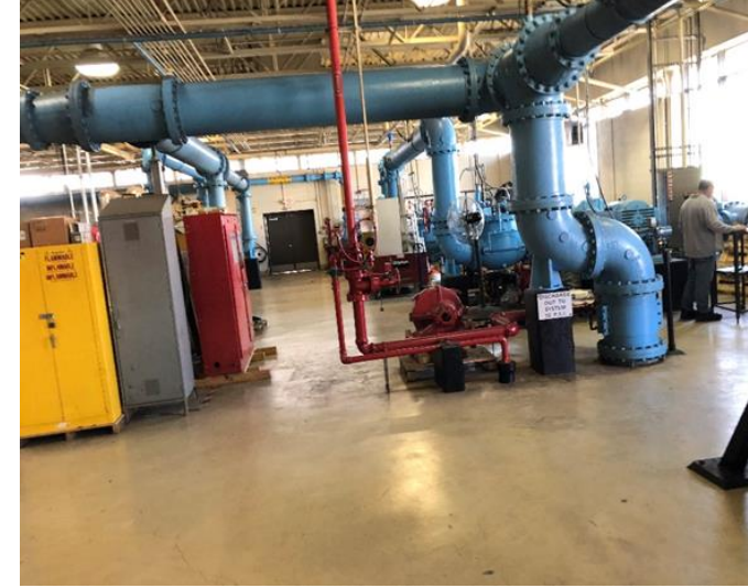
Photo 1 – Mechanical Fire Protection
