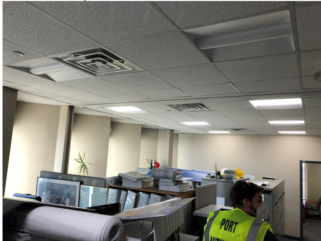
Mechanical Fire Protection Fig 08
