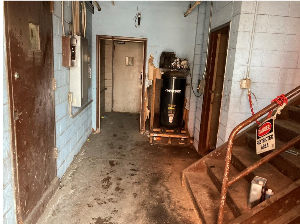
Mechanical Fire Protection Fig 11
