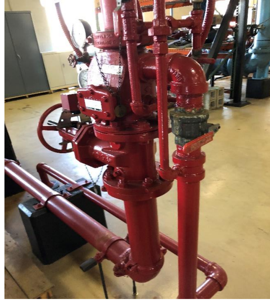
Photo3 – Mechanical Fire Protection – Alarm Check Valve Serving Sprinkler System
