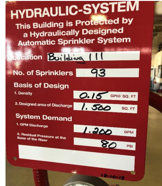
Photo 2 – Mechanical Fire Protection
