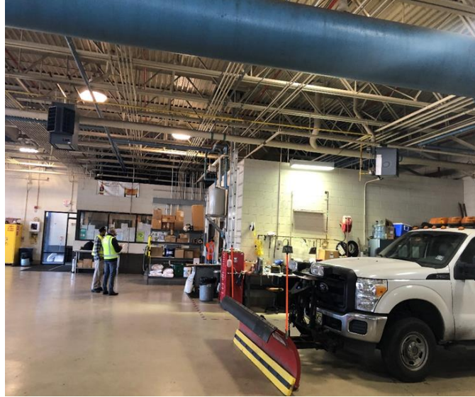
Photo 1 – Mechanical HVAC – Ceiling Mounted Unit Heaters
