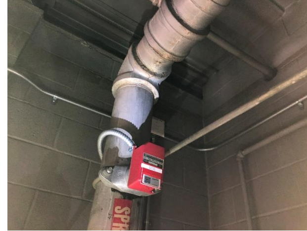
Mechanical Fire Protection Fig 03
